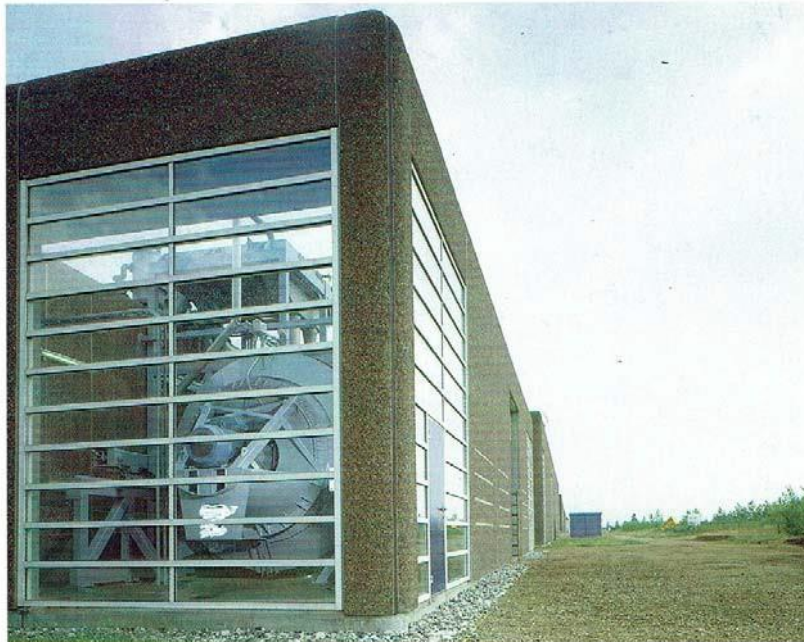
System installed at Lego System A/S chilling water from approximately 13.5°C to 9°C
